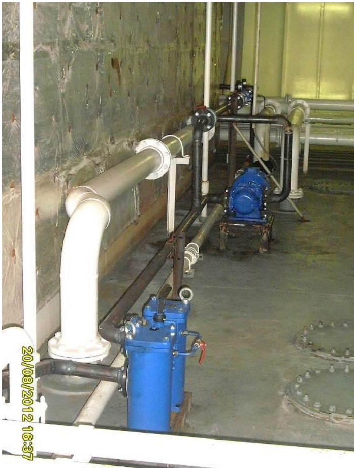
Module TRGA on the settling tank on 20 August 2012
