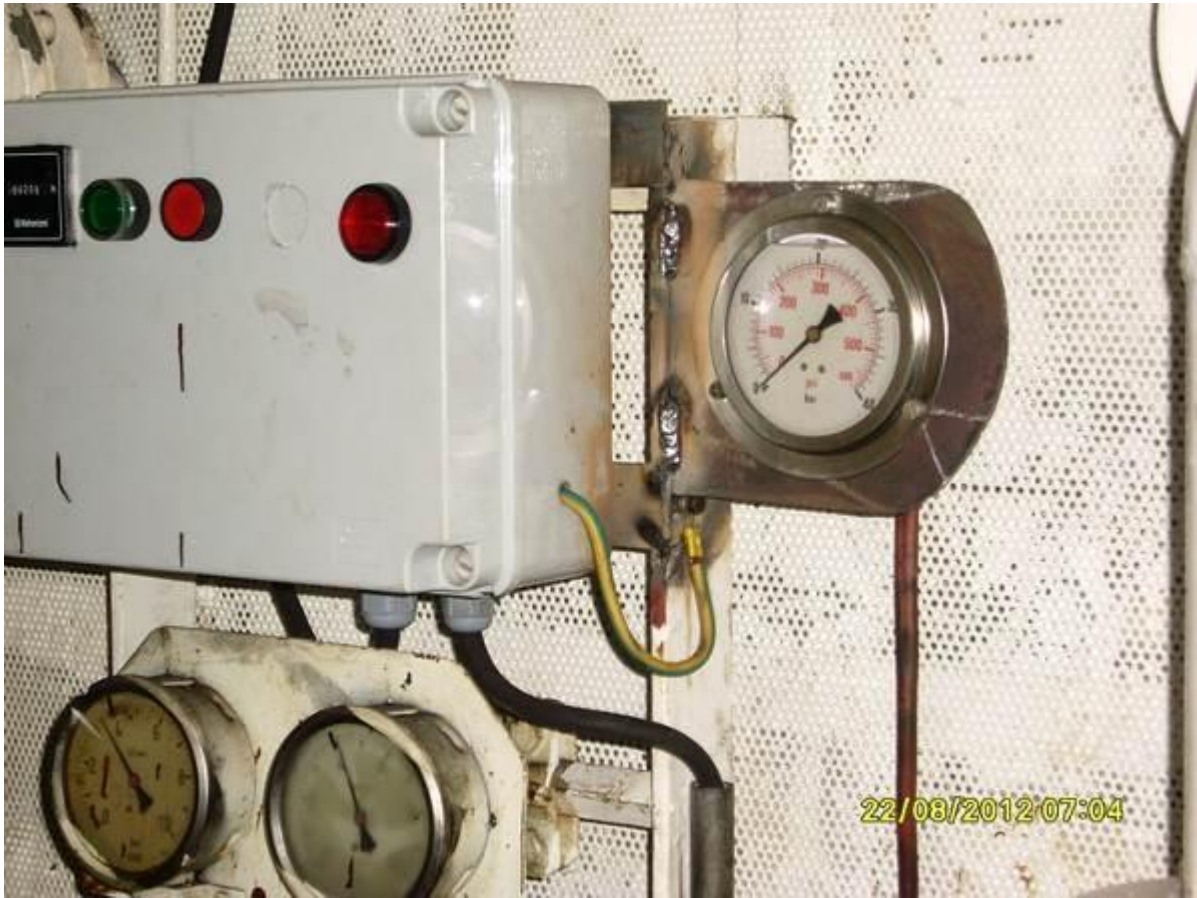
The Module TRGA switched OFF on the buffer tank
