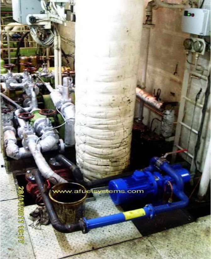
Installed Module TRGA on the buffer tank on 28 November 2011
