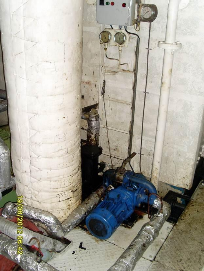
Module TRGA on the buffer tank on 19 August 2012
